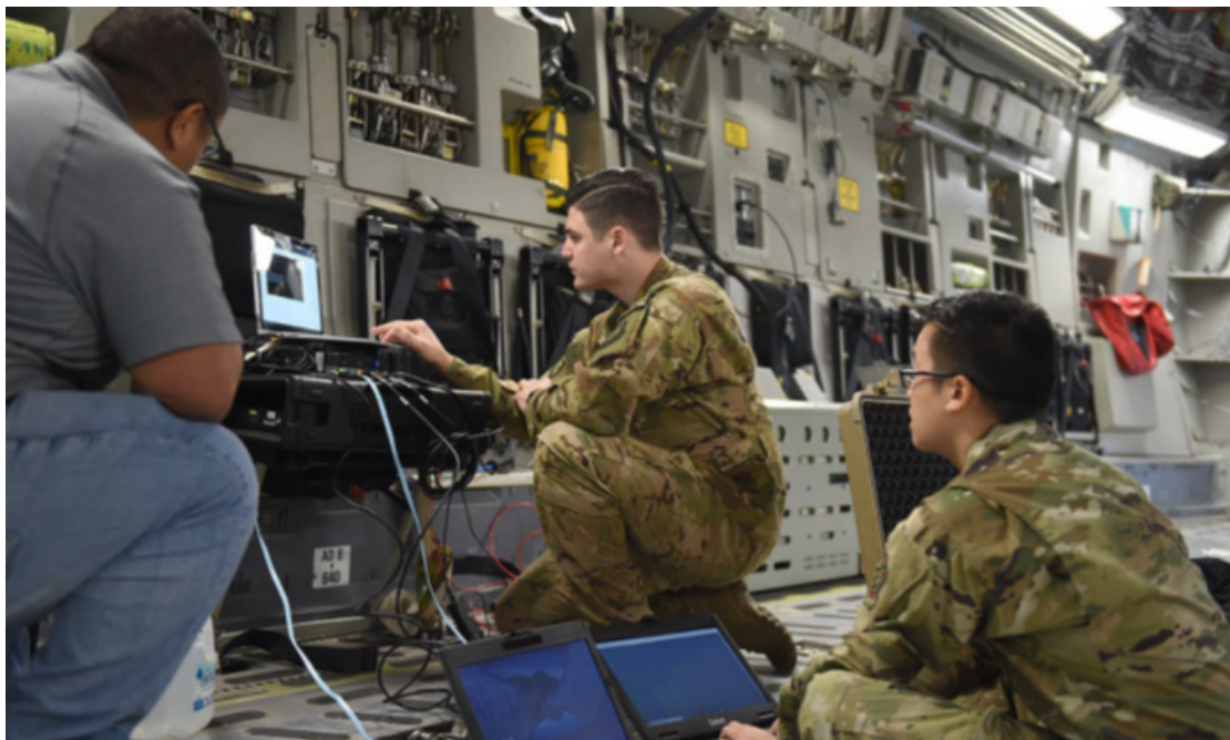
Figure 2: A DOD contractor, 1st Airlift Squadron communications systems operator, and Air Mobility Command cyber transport systems technician, test a fixed installation satellite antenna (FISA) connection onboard a C-17 Globemaster III on Joint Base Lewis-McChord, Wash., June 5 2020. The FISA was set up to work with a dynamic re-tasking capability (DRC) system, enabling higher connection speeds and more efficient communication between the aircraft and the ground.
